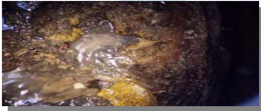
Grease buildup in a sanitary sewer!
