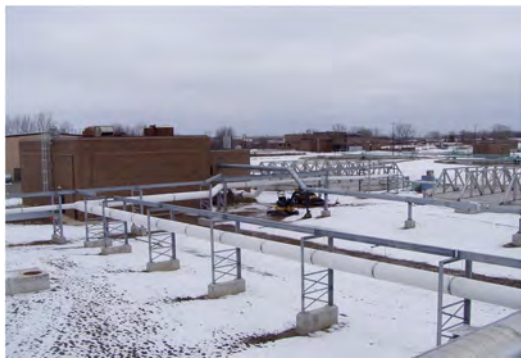
View of Phase II Odor Control Ductwork
