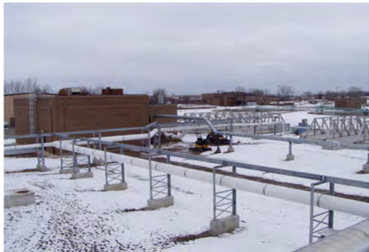
View of Phase II Odor Control Ductwork
